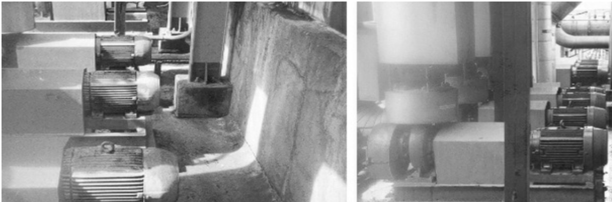
Figure 11. Cold water pumps - Group 1
